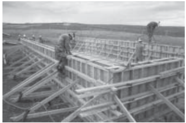
Figure 23a. 864th Combat Engineers from the Presido constructing 4'-9" wing-wall forms preparatory to pouring concrete.
