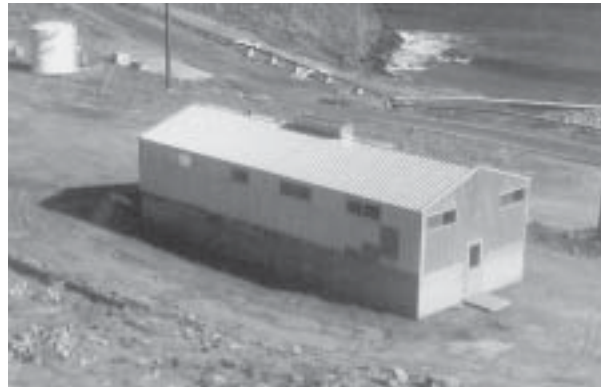
Figure 23c. The 20' x 49-6" Pascoe building is fully assembled awaiting an epoxy-based paint coating. Total time for construction: 11 days. Total cost: $12,000.
