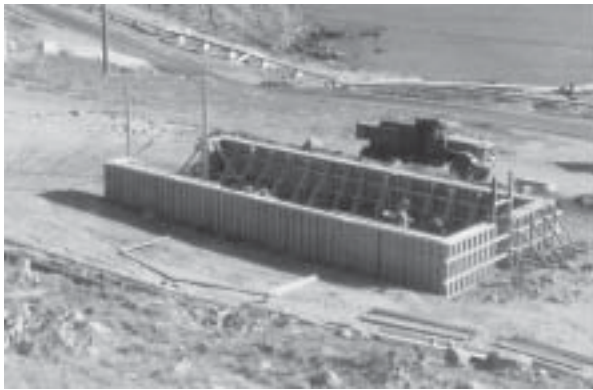
Figure 23b. Wing-walls pouring completed. When forms are removed, the Pascoe building kit is assembled on this elevated foundation.
